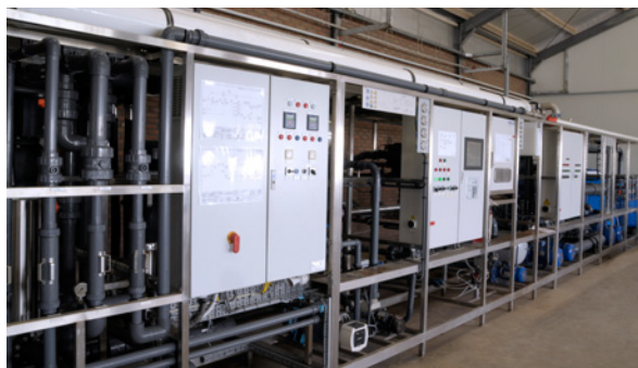
Figure 11. Picture of the technical installations in the water technical room. The setup shown here allows the grower to quickly check the proper functioning of all systems.
